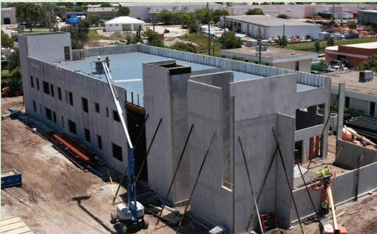
Construction at The Lord's Place new Australian Campus. Photo Credit: Tracey Benson Photography.
